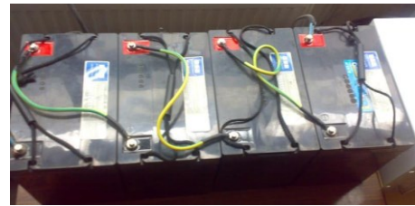
Fig. 4. Acumulatori Solar Series 12V /150 A.
